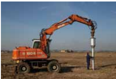
Easy Installation of the Borefundaments. Simple Drilling in with a hydraulic excavator
